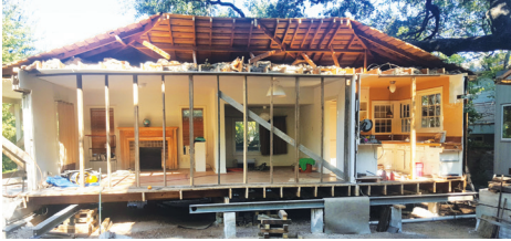
A house is cut in half and temporary wood supports installed to prepare for relocation. (Credit: Kathy Robinson)
