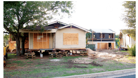
A pair of Duval Avenue bungalows, owned by a University of Texas at Austin fraternity and scheduled for demolition, were sold and relocated to two adjacent lots in the JJ Seabrook Neighborhood. Two 1930s Bergstrom Air Force Base barracks, previously moved to the lots in the 1940s, were also relocated on-site and lifted to become garage apartments. The bungalows and barracks received full renovations, orchestrated and designed by Architect Ben and Sandi Heimsath. (Credits: Ben and Sandi Heimsath)
