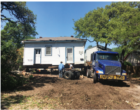
A 1933 main house approved for demolition was purchased by a general contractor and relocated outside of Austin. The porch, which extends the entire length of the front facade, was temporarily removed for transport. (Credit: Sarah Gamble)
