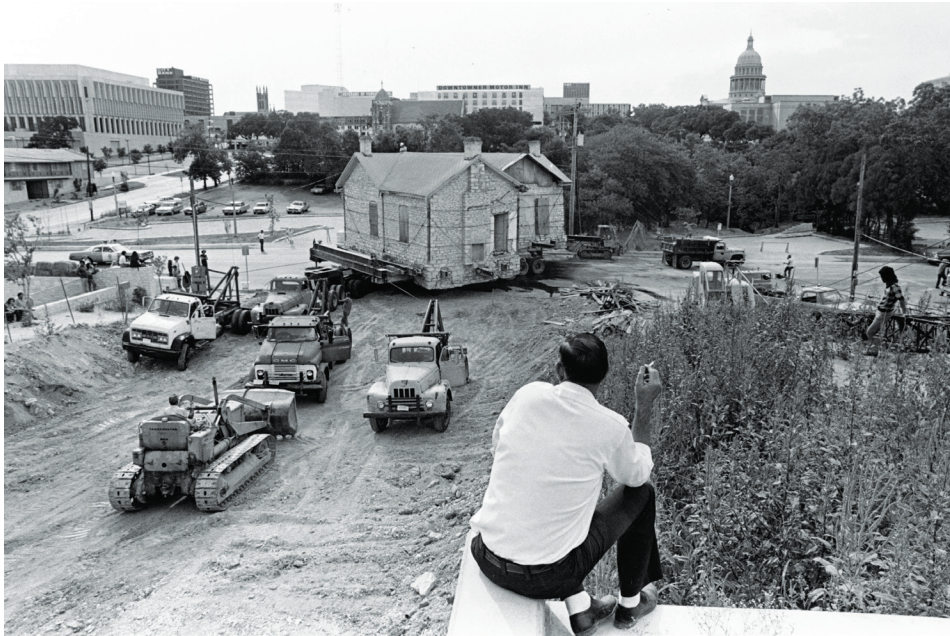
The William P. Hardeman House is relocated from 401 East 16th Street to 1111 Red River Street to become part of downtown Austin's Symphony Square. (Credit: PICH-03525, Austin History Center, Austin Public Library)
