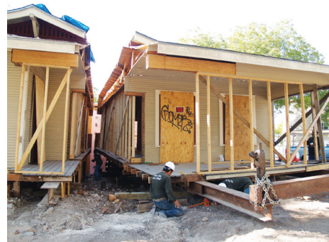
A bungalow is cut and lifted on temporary steel rails in preparation for relocation. (Credits: Ben and Sandi Heimsath)
