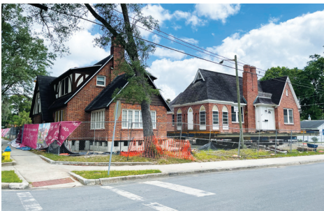
Contributing to a local historic district, two Tudor Revival houses on opposite sides of a block in Gainesville, Florida were relocated to make way for a new sorority house near the University of Florida. Temporary steel rails were inserted through the skirt to lift and support the hybrid structures with their brick façades and wood-framed interiors. (Credits: Carly Walker, Sarah Gamble)
