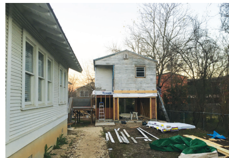
Built in 1937, a garage apartment was lowered, relocated and rotated 180 degrees, then lifted for reuse. In addition to a new exterior stair and one-car garage below, the interior renovation preserved the art deco details, pine flooring, and cabinetry, while adding a new bathroom, HVAC system, and plumbing. (Credits: Sarah Gamble)
