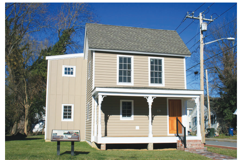
The Buffalo Soldier House in Easton, Maryland's Hill Neighborhood was slid 8 feet horizontally on steel rails using manpower and soap. Built circa 1869, the house was pushed away from modern power lines and the adjacent roadway, in preparation for a full rehabilitation designed by Encore Sustainable Architects and sale as an affordable home for a military veteran. (Credits: W. Ward Bucher, AIA)
